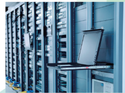
Control Room/ Data Center
